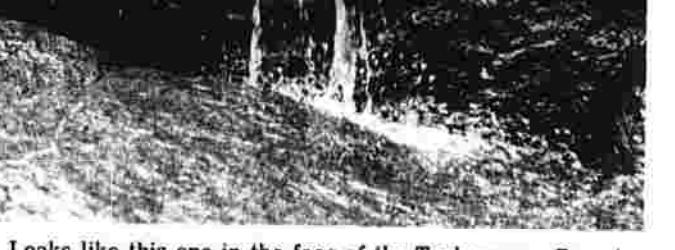
Leaks like this one in the face of the Tankeroosan Dam in Vernon hint at the force of the water behind it. (Herald photo by Strempler)
