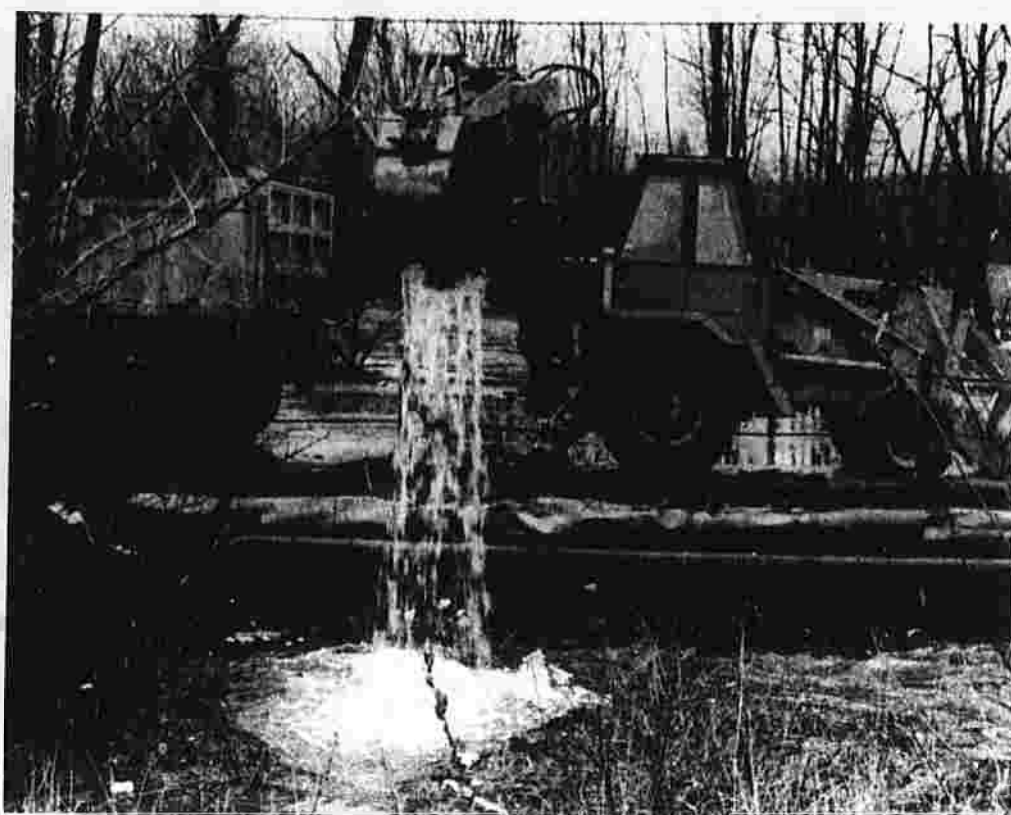
Town crews removed debris from the upstream side of the Adams Street bridge over the Hockanum River in Manchester. (Herald photo by Pinto)
